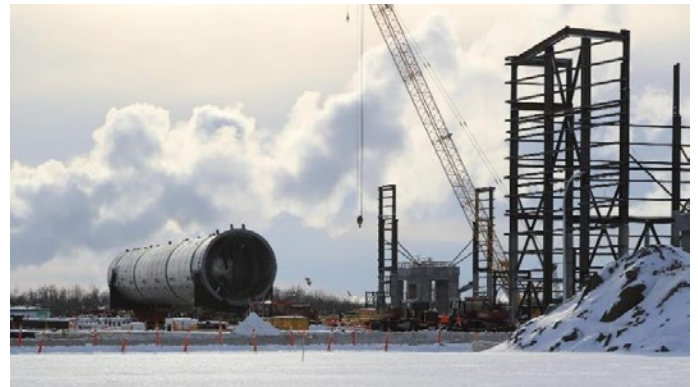
Propylene-Propane Splitter for the Complex
